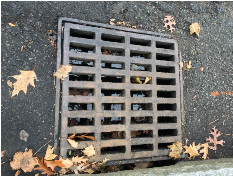
This catch basin was found full of water due to a clogged drain pipe
