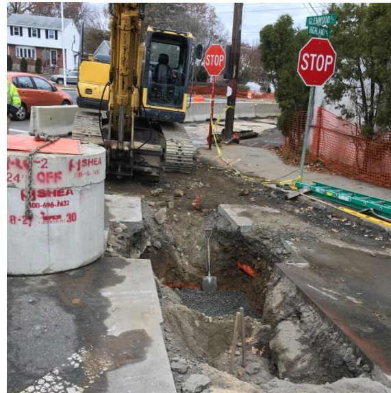
The crew is preparing to install a new catch basin, which will be placed at the center of the photo
