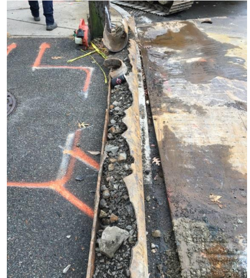
Broken drain pipe full of debris
